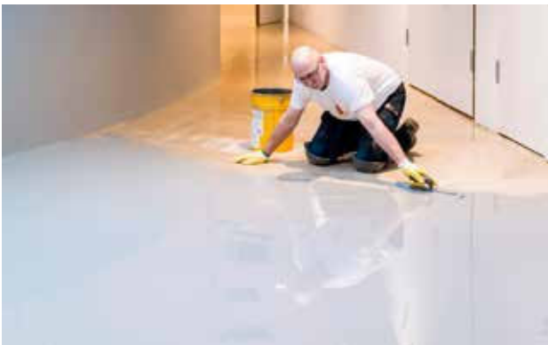
STEP 3. Self-leveling materials are applied in one or several layers to create a seamless base. Experts will pour and distribute the liquid material by using special squeegees, hand trowels, stand-up trowels and spike rollers in the process to assure a perfectly even and smooth surface.
