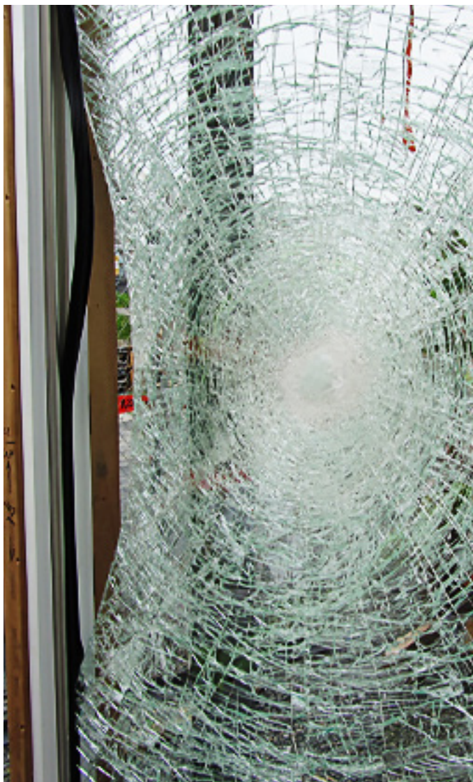
Window System Failure
