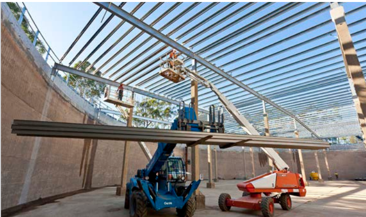
ZAM® purlins used for roofing of water reservoir
